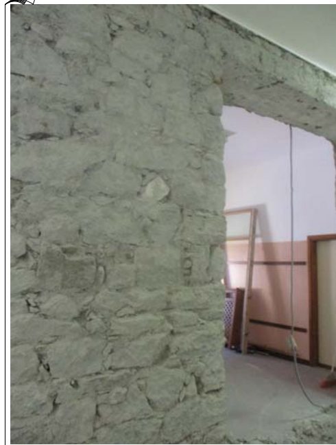
Dettaglio fessurazione architrave. by Arch. Sergio Ghirardelli (DL)
