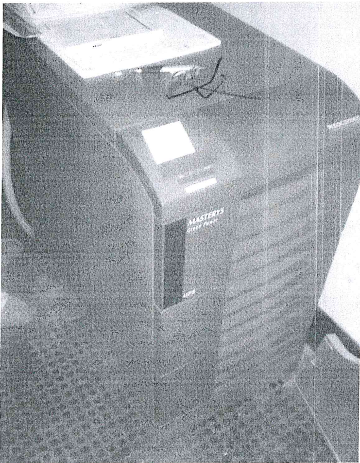
UPS SOCOMEC 30 Kva
